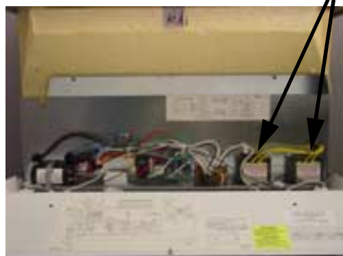
FIGURE 30. Electrical Box 2XX Dual Transformer
